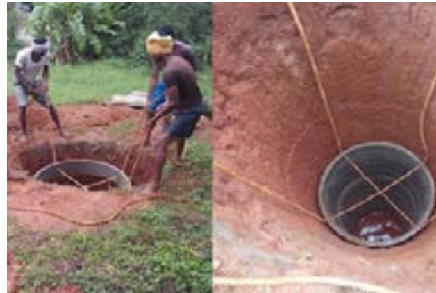
A new open well in the community
